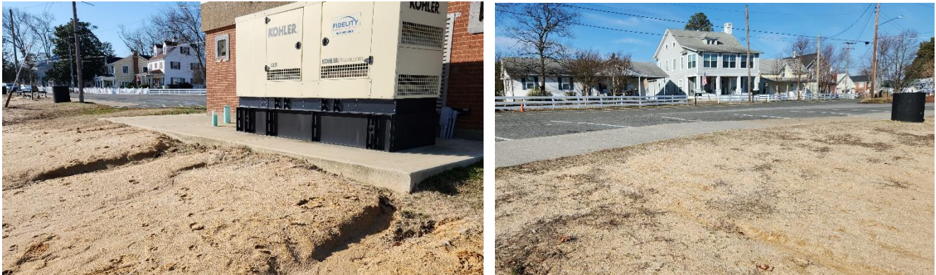
Figure 2-12: Beach erosion from generator platform, bathhouse/bathroom, and parking/pavement (February 1, 2024)
