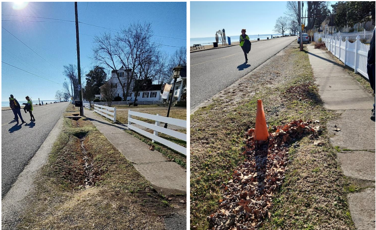
Figure 2-16: Opportunity for bioretention swales and stormwater infrastructure upgrades on the west side of Irving Avenue (February 1, 2024)
