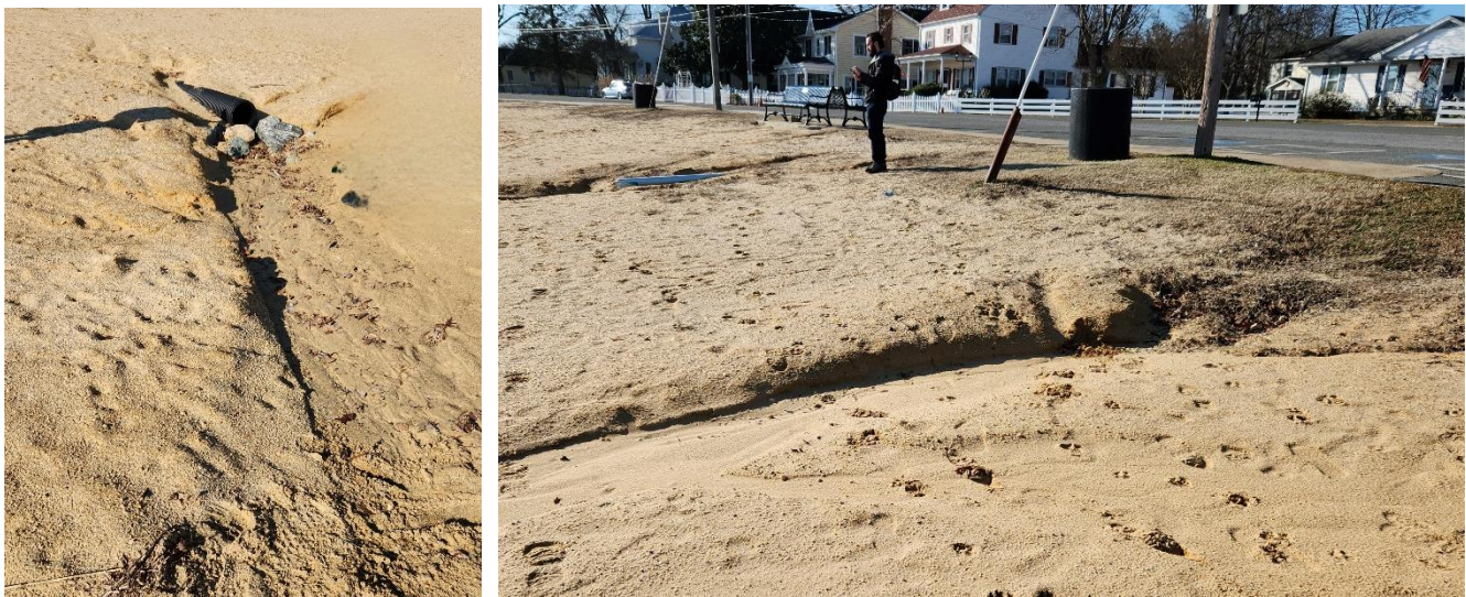
Figure 2-7: Beach scouring at an outfall (left) and from pavement (right) along Beach Terrace/Irving Avenue (February 1, 2024)
