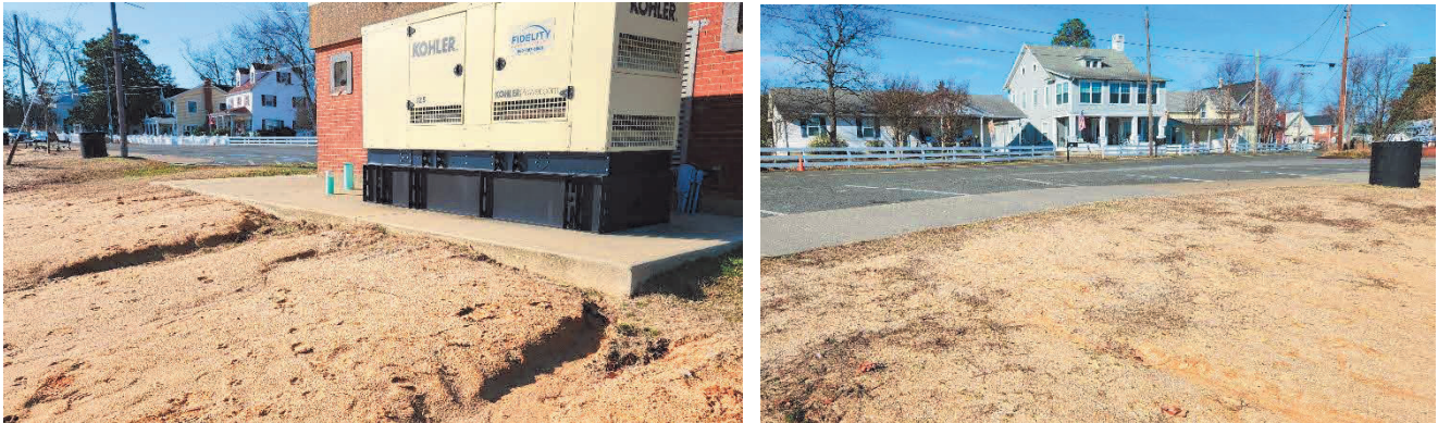
Figure 2-8: Beach erosion from generator platform, bathhouse/bathroom, and parking/pavement (February 1, 2024)
