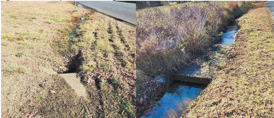
Figure 2-5: Examples of standing water in the Dennison Street area
