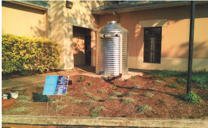
Figure 2-13: Example of a roof leader cistern
