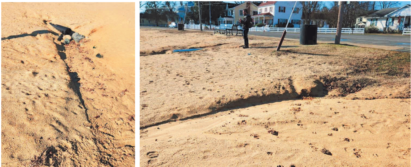
Figure 2-7: Beach scouring at an outfall (left) and from pavement (right) along Beach Terrace/Irving Avenue (February 1, 2024)
