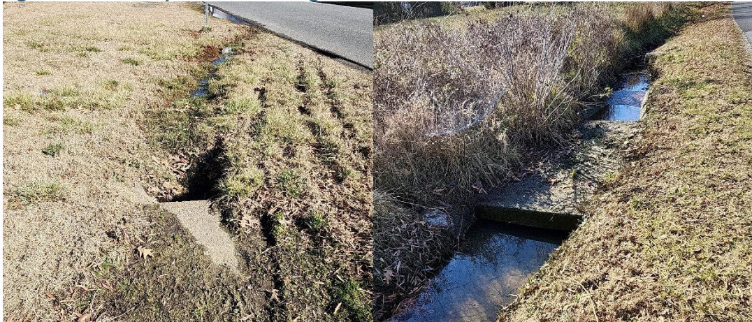
Figure 2-6: Examples of standing water in the Dennison Street area
