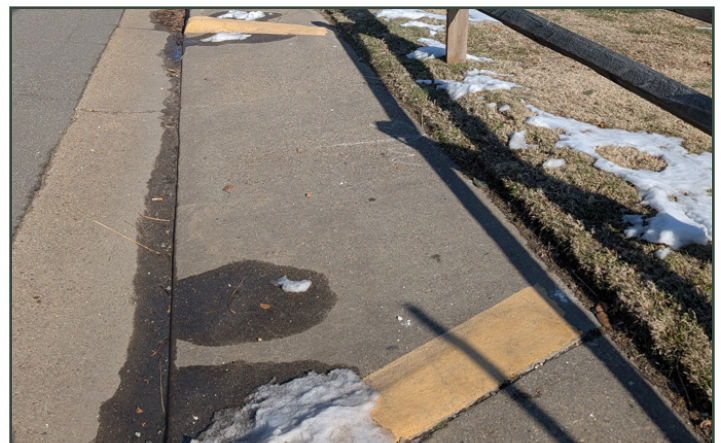
Figure 12. Curb cut leading to a non-existent driveway at Town Hill.
